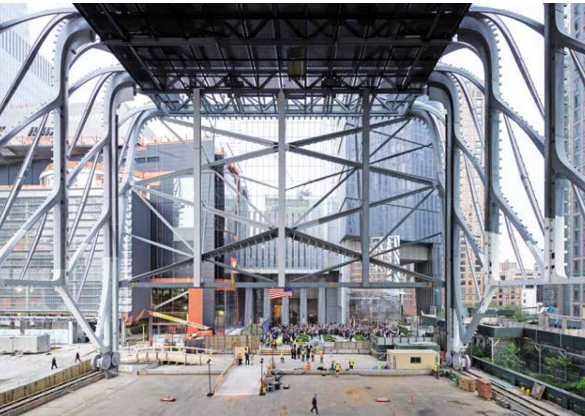
Construction view of Diller Scofidio + Renfro's the Shed, anticipated completion 2019, New York. Photo: Iwan Baan.
